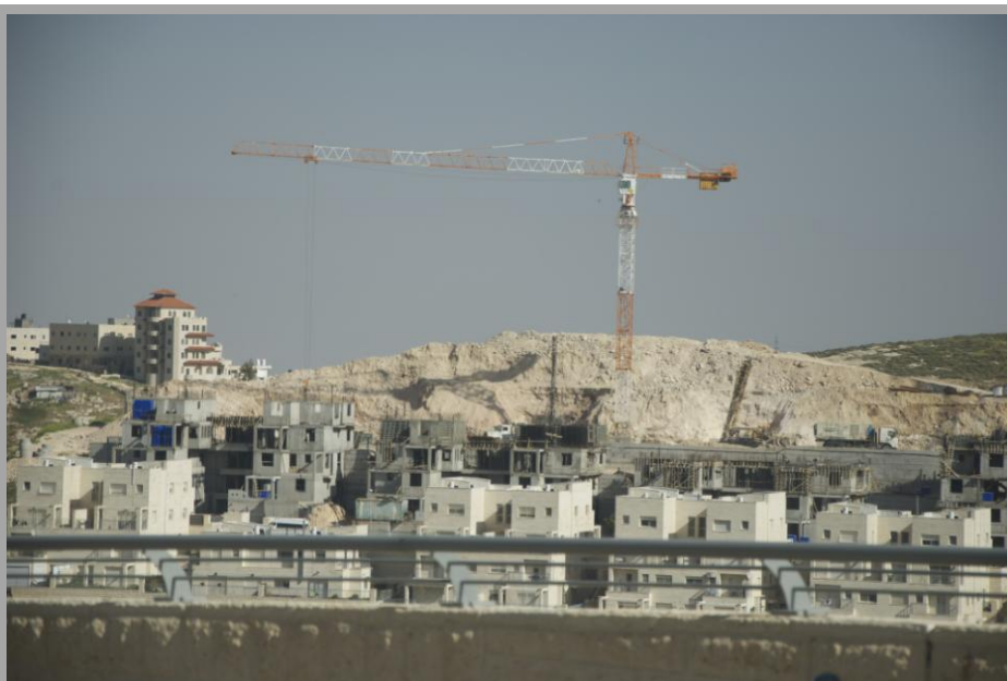
Many Palestinians are employed in constructing the vast settlements that dominate the West Bank
